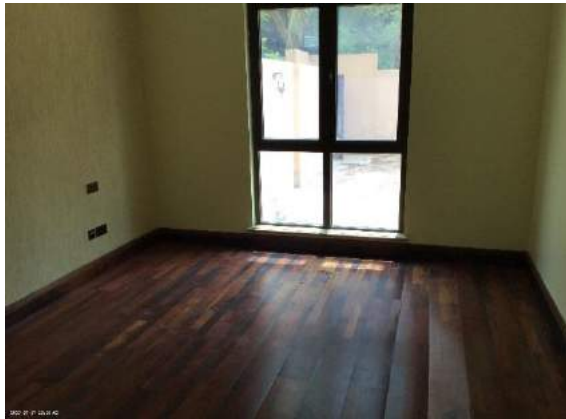
Bedroom with Damaged Flooring
