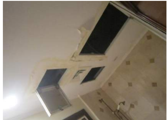
Evidence of Water Leak in Bathroom
